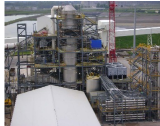
AEP Mountaineer USA - 58 MW th Chilled Ammonia - Kohle
