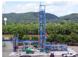
Dow Chemical Co. USA, West Virginia Advanced Amine
